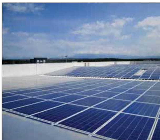
View of panels arranged on the roof of a shopping center
