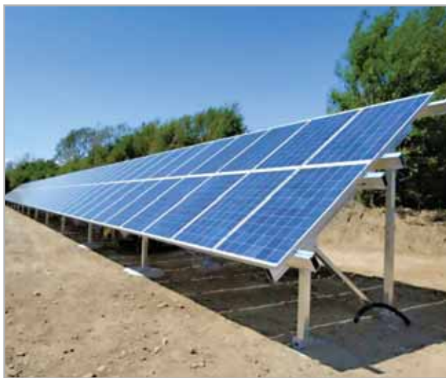
Ground mounted solar panels
